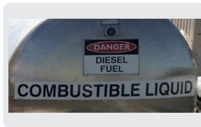
Aboveground Diesel Tank
